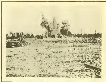
Quarrying limestone in Onandaga County; 2,000 pounds of dynamite were exploded in this shot.
